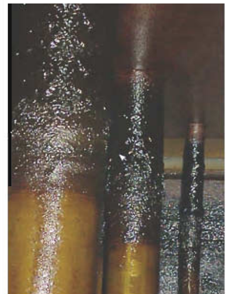
Figure 1. An advanced case of deposits accumulating on metal surfaces above the oil level
