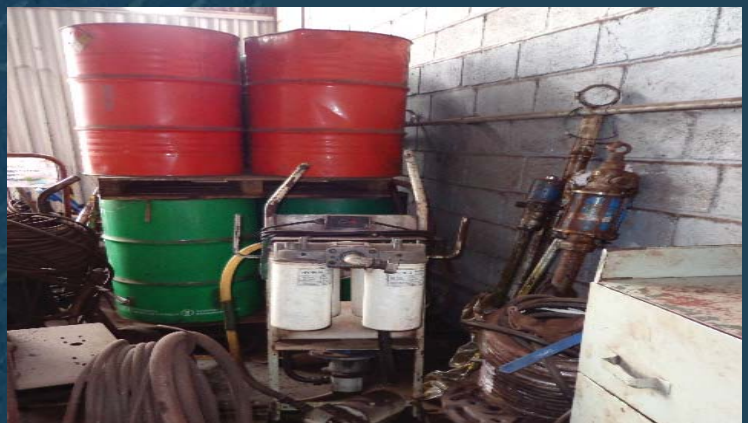
Before the improvements were made, only one filter cart was used to filter all types of lubricants.
