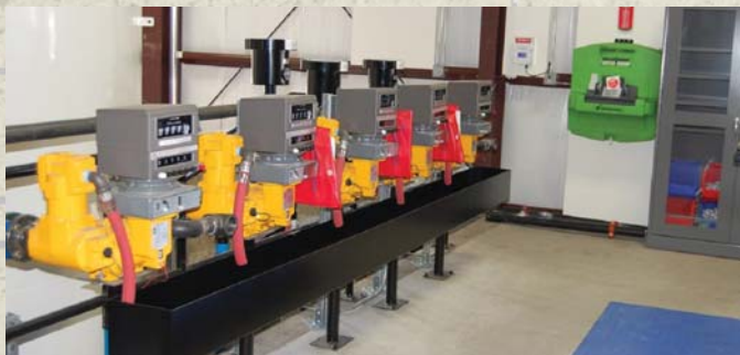
All bulk and packaged lubricants are dispensed utilizing temperature-corrected flow meters.
