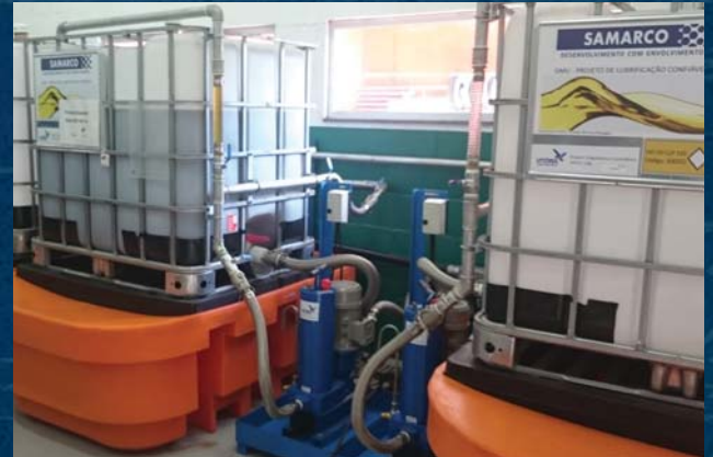
New oil is pumped through hard piping to the treatment room.
