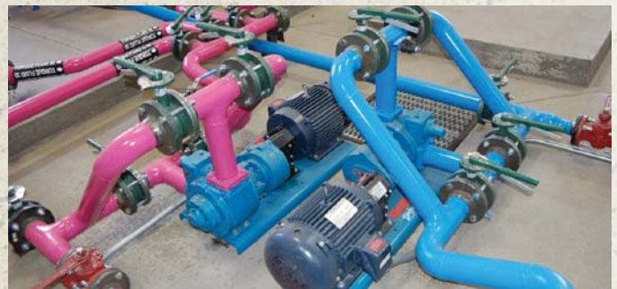
The piping for each tank is painted in accordance with the product color-identification policy.
