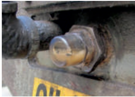
Figure 4: Sight glass revealing cloudy oil.
