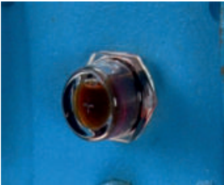
Figure 1: Sight glass indicating oil level is too high.
