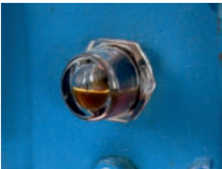
Figure 3: Sight glass indicating oil is at the appropriate level.
