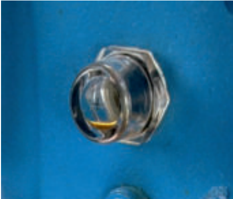
Figure 2: Sight glass indicating oil level is too low.
