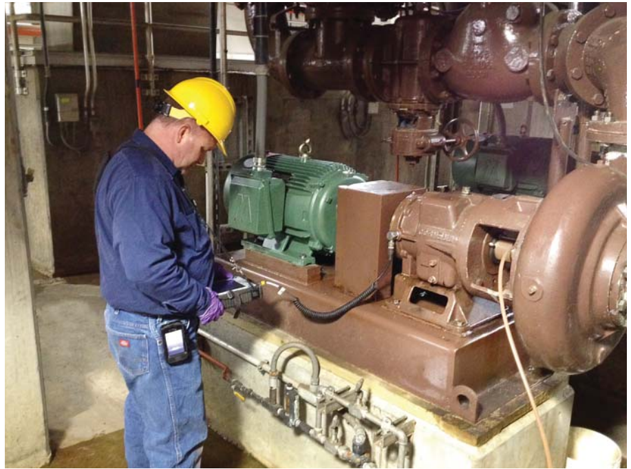
In a two-tiered predictive maintenance program, a skilled PdM team with sophisticated data-collection hardware and analysis software supports and collaborates with maintenance crews equipped with simpler tools for detecting problems in their plants.
