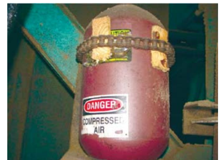
Figure 5. A mislabeled accumulator
