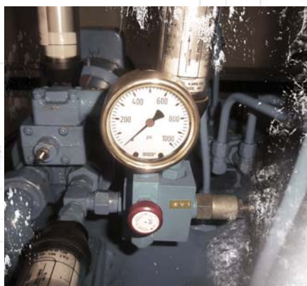
Most systems have a dump valve that allows high-pressure fluid in the accumulator to dump to the tank, permitting the pressure to drop to zero.
