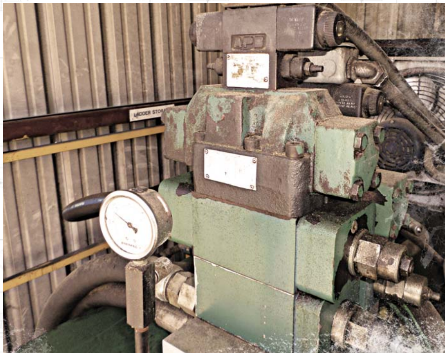
This image shows a tilt hoist with a failed main directional valve.
