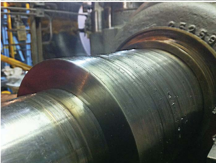
Pump shaft damage
