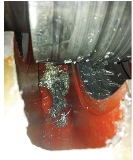
Pump casing oil drain
