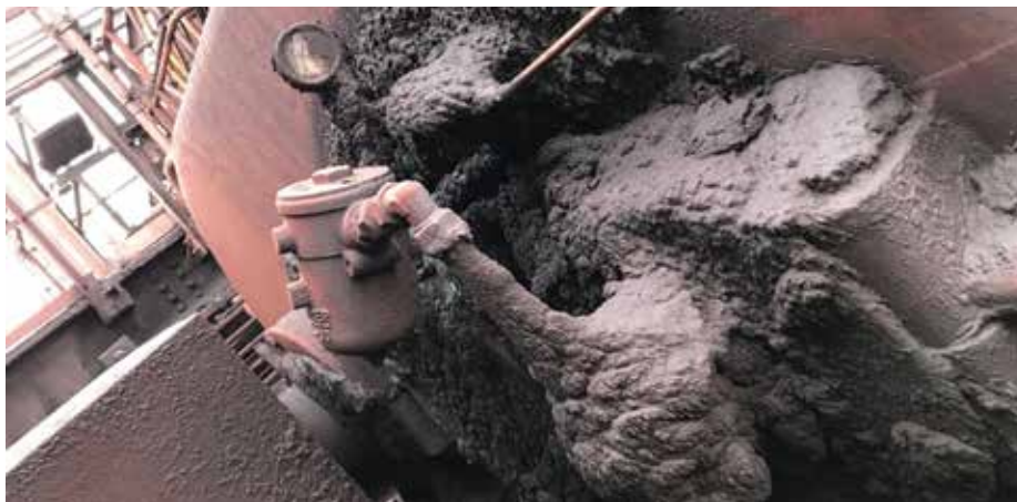
Figure 4. Large gearbox (4 reduction stages) used in a steel mill. Leakage around oil pump went unnoticed, ignored or just deferred for later repair. Little by little the gearbox drained of oil resulting in a thick dust cake. Oil pressure gauge was obstructed by the cake. Ref. Ronald van Druuten
