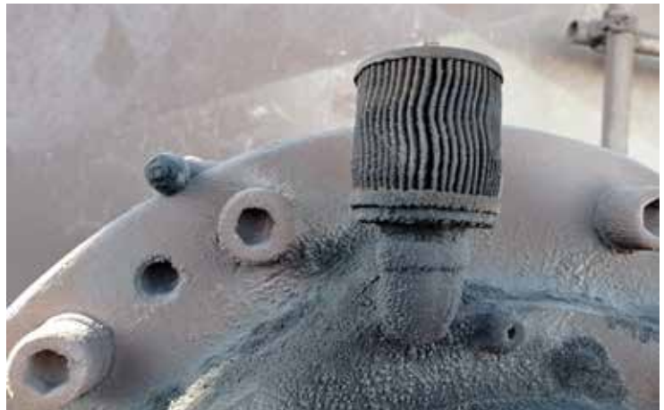
Figure 1. Backstop breather has caked-on dirt down the elbow and along the case. This is usually due to oil mist that has migrated out of the headspace and collected on nearby surfaces. Airborne particles adhere and build up on the oil-damp surface forming layers of heavy, caky grime. Too much oil mist results in the need for frequent top-ups (oil and labor costs) and fluctuating oil level control. In many cases breathers function much better and last longer if they are positioned higher with a pipe extension. Ref. Kevin Albert
