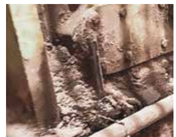
Figure 3. Dust cake buildup near leak area on gear case and base. Notice sight glass and oil fill port. Ref. Torki Ibrahim
