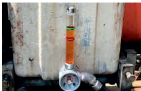
Figure 3: A columnar level gauge installed at the proper level.
