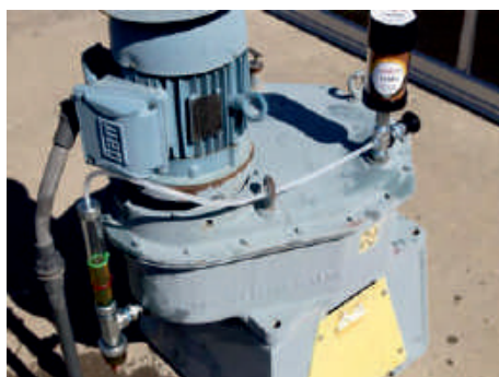
Figure 2: A columnar level gauge installed with a desiccant breather.
