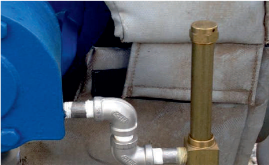
Figure 6: The bends in this pipe will trap oil in the gauge.
