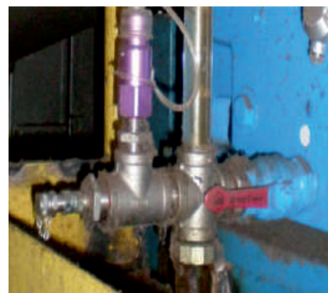
Figure 4: A columnar level gauge with a shut-off valve.
