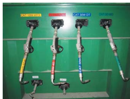
Dispensing nozzles are now labeled and color-coded.
