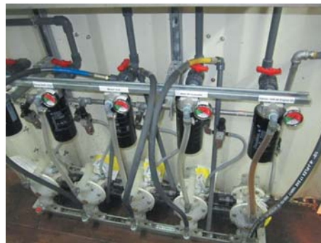
New oil is filtered when it is transferred into the storage tanks and then again upon dispensing to ensure the cleanest oil goes into the equipment.
